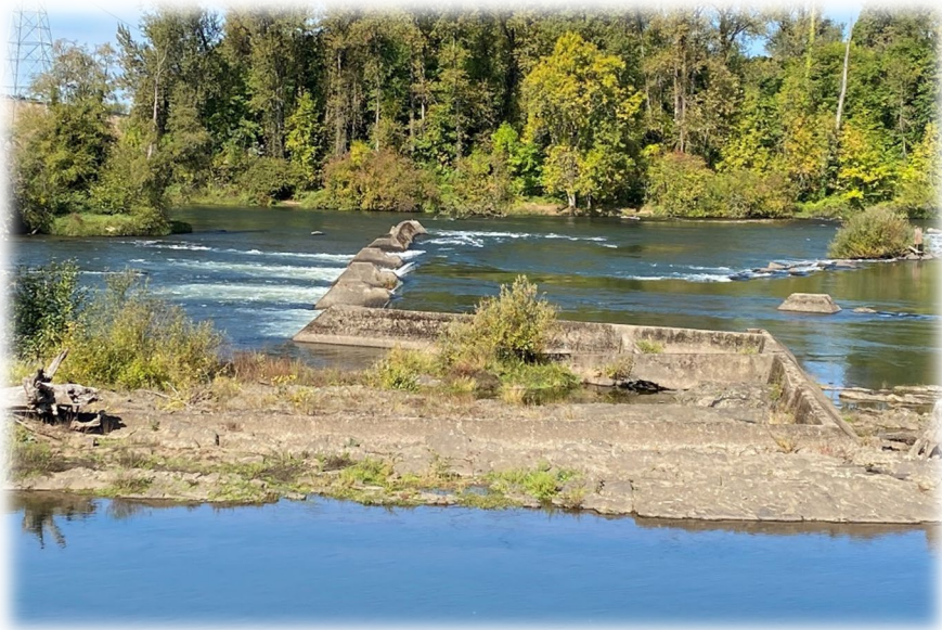
Willamette River mill dam ruins viewed from river left
